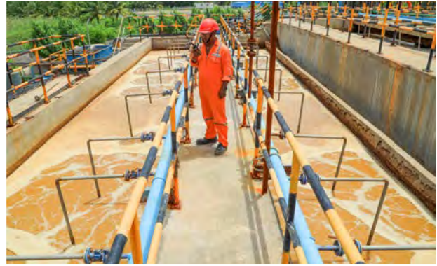
Effluent Treatment Plant
